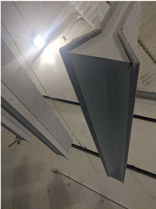
Figure 4 – Lens exposed at underside
